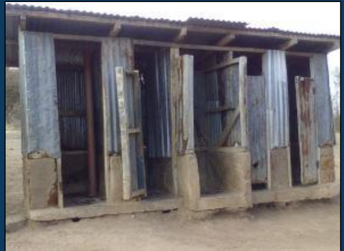
One of two existing latrine blocks serving 475 pupils. Two blocks of 8 latrines each will be built.
