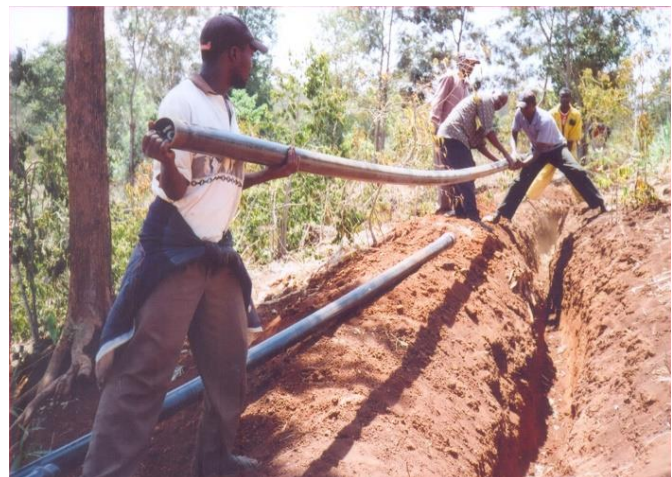
Laying pipes to supply water from the river to the water tank
