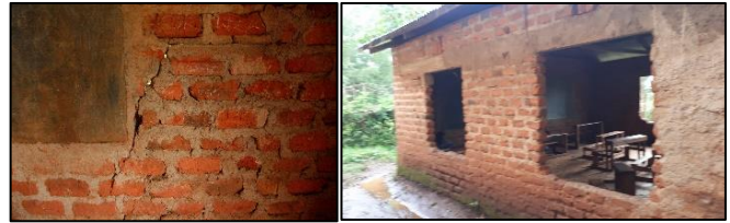
Cracks in the wall and unfinished construction
